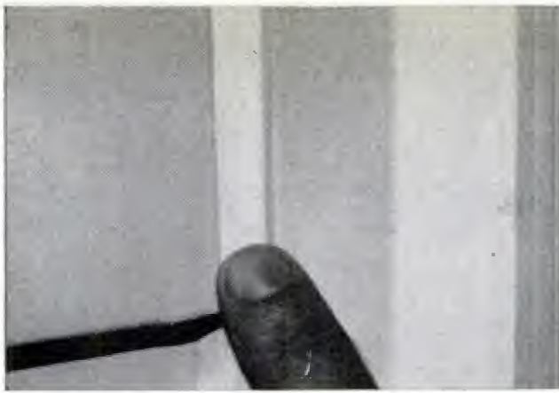
ACRYLIC-CAULKED JOINT between end of siding and trim is in good condition after two years' exposure
